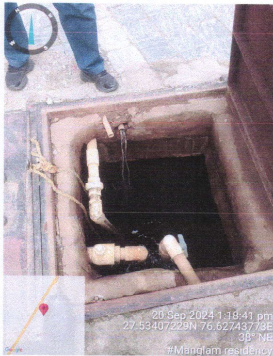
Figure 4: Photograph of water storage tank in Manglam Residency.
